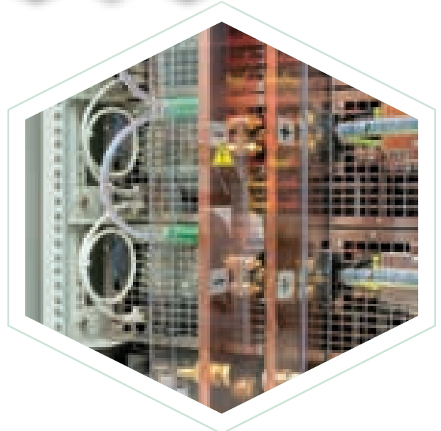
DC output via copper rails (DC bus) AC input selectively fused Interfaces integrated.
